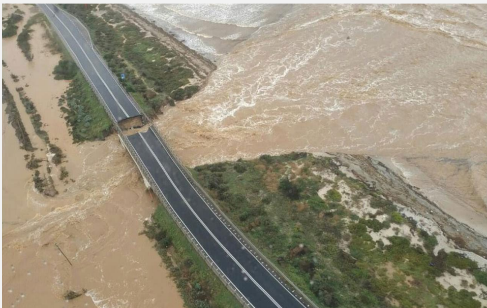
Collapse of the bridge along State Road 195 over the Santa Lucia River (Cagliari, Italy). Source: La Repubblica, 2018.
