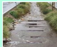
Bioretention systems (vegetated drains, etc.)
