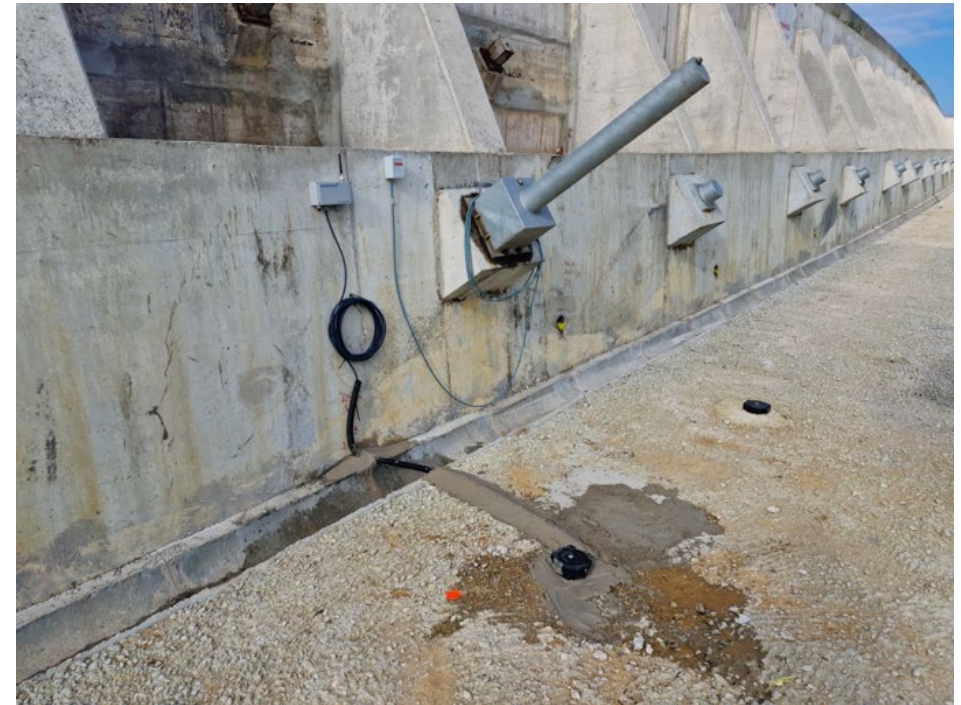
WR LOG Wireless Monitoring System
